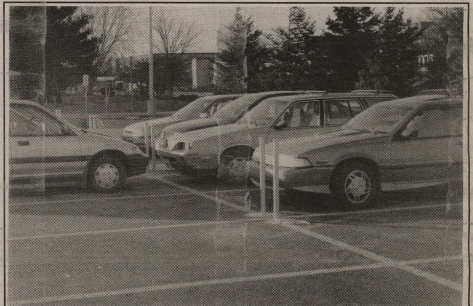
Posts are installed in Lot X and meters will be ready by spring. The meters will replace the current draw gate system. (Photo by Cody Strathe)
