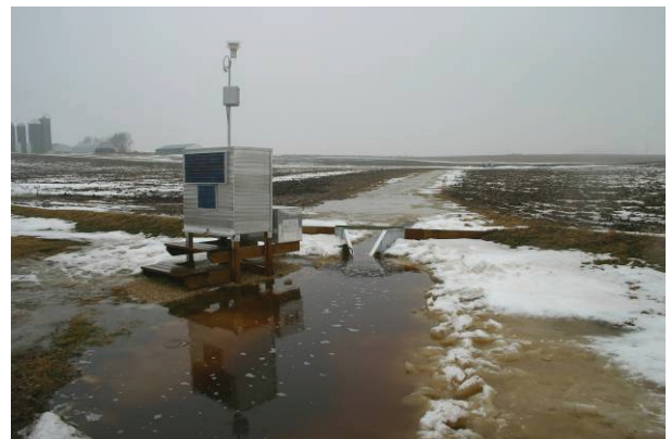
In 2004, the culvert downstream of S7 was not properly cleared of snow.
